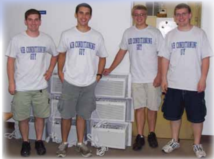
Four seminarians are helping install air conditioners this summer. From left to right: Curt Vogel, Andy Mattingly, Alex Kreidler, and Josh Barlett. The "Air Conditioning Guy" t-shirt readily identifies them when they show up at an elderly person's door.
